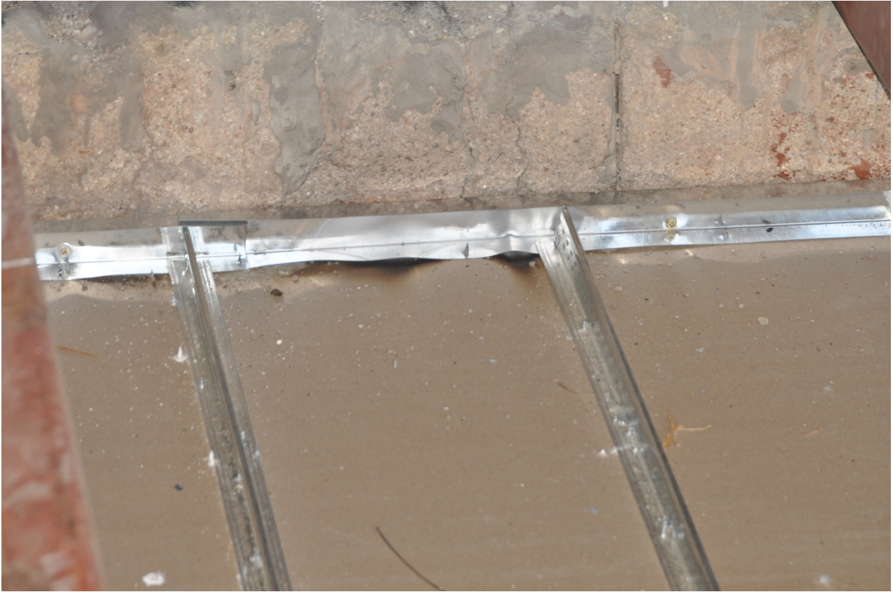
Figure 3.3: Charring and slight buckling of the perimeter fixing
