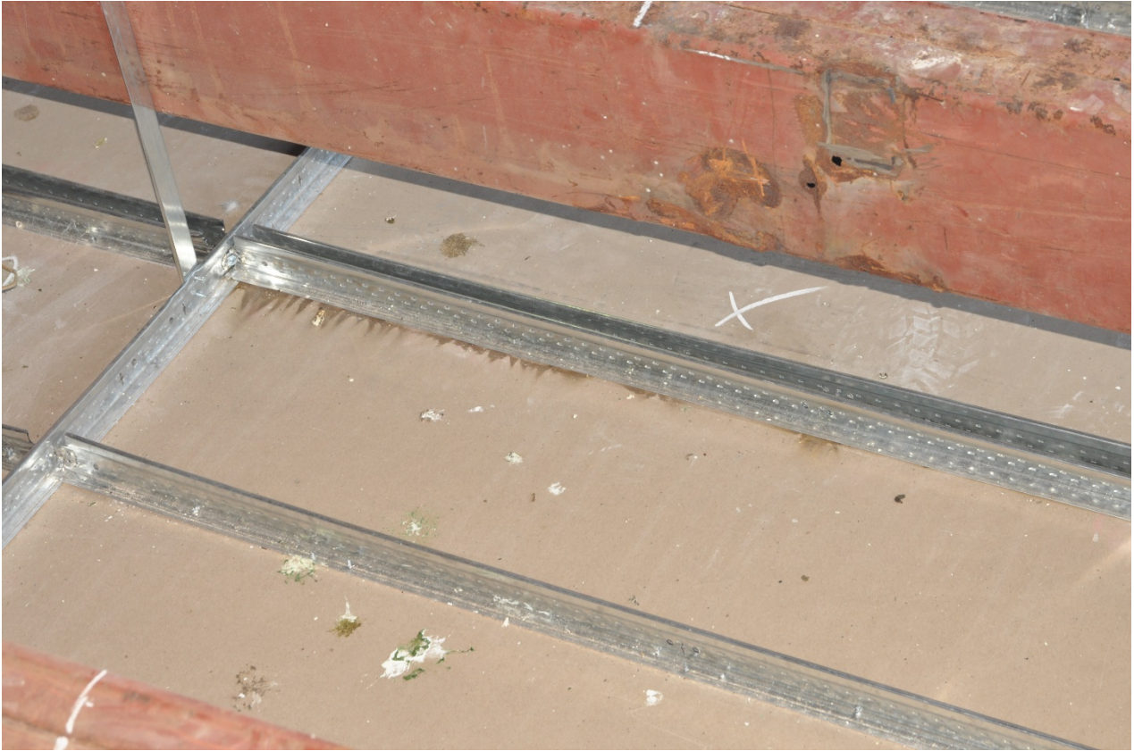
Figure 3.7: Discolouration visible (mid-section joint of specimen)
