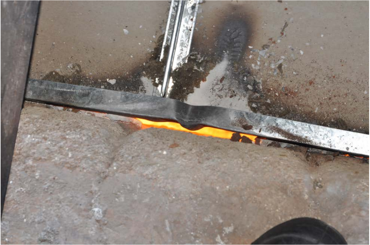
Figure 3.5: Edging buckling and board charring
