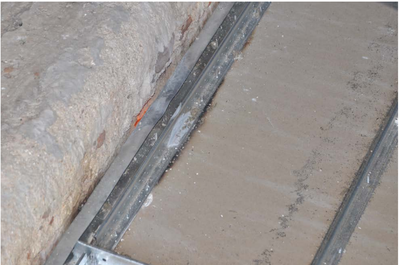
Figure 3.6: Charring at front perimeter
