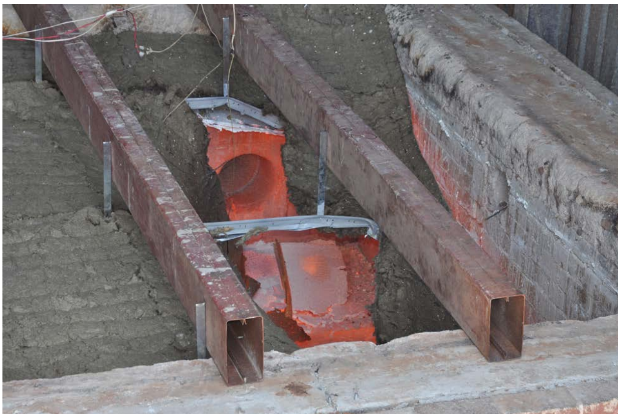
Figure 3.9: System collapsed near back perimeter
