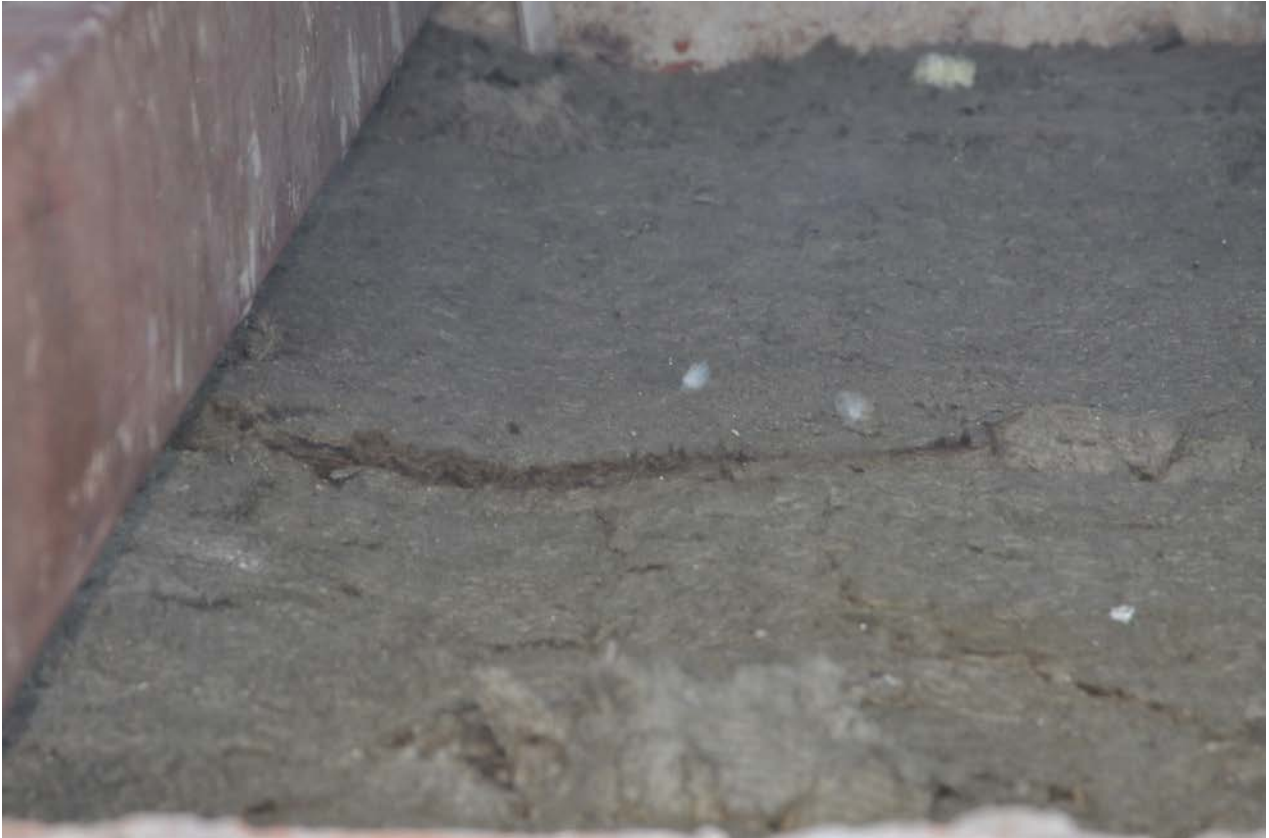
Figure 3.5: Insulation darkening on joint
