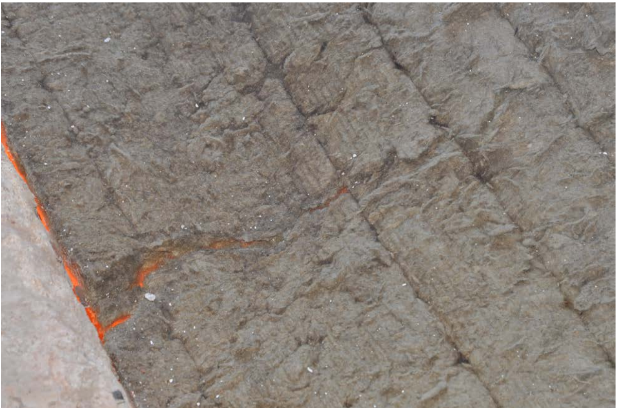
Figure 3.8: Glowing observed through insulation
