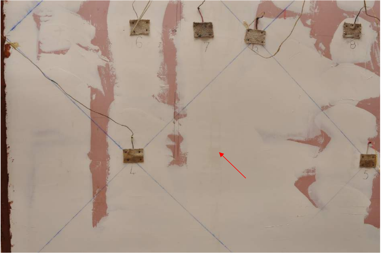
Figure 3.4: Slight discolouration on LHH
