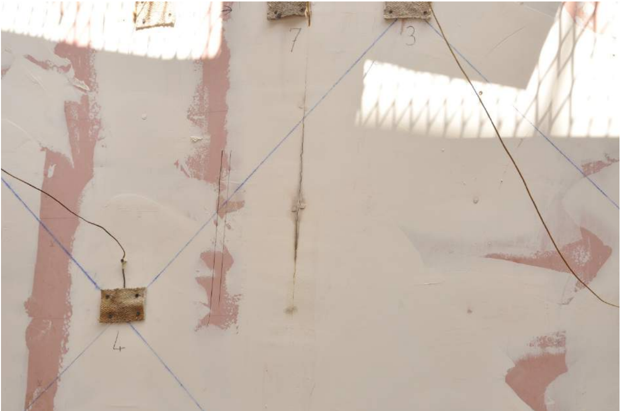
Figure 3.8: Crack discolour on LHJ
